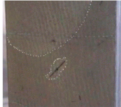
Fig. 1: Debonding of composite patch from cracked aluminium panel
